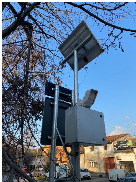
Figure 3: Solar powered traffic sign battery case
